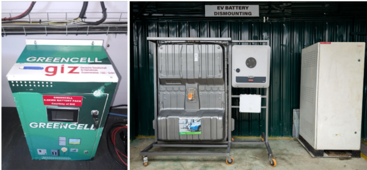
a) 6.8kWh "Greencell" pilot repurposed battery using Gen 1 Nissan LEAF EV battery modules b) 7.7kWh repurposed storage solution with original battery pack form factor with inverter
